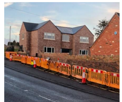
A dangerously uneven pavement on Bromsgrove Road. Reported and repaired.
